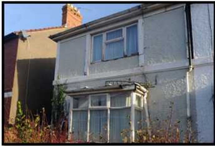
Left to rot: The house has been empty for 17 years
