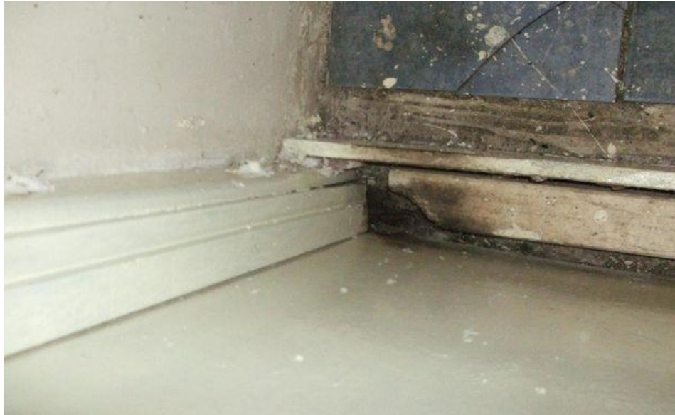
The Mansel Street takeaway's preparation area was also found to be caked in dirt and grease (Photo: Wales News Service)
